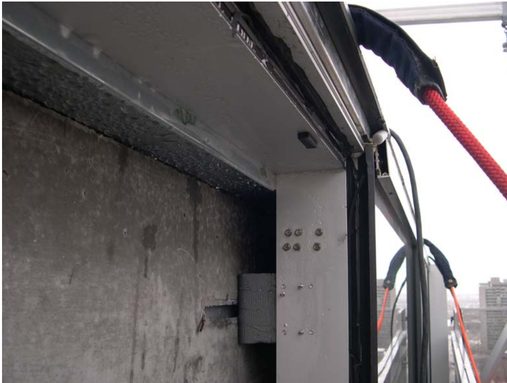
Figure 1: Condensation on curtain wall components behind insulated spandrel panel assembly.
