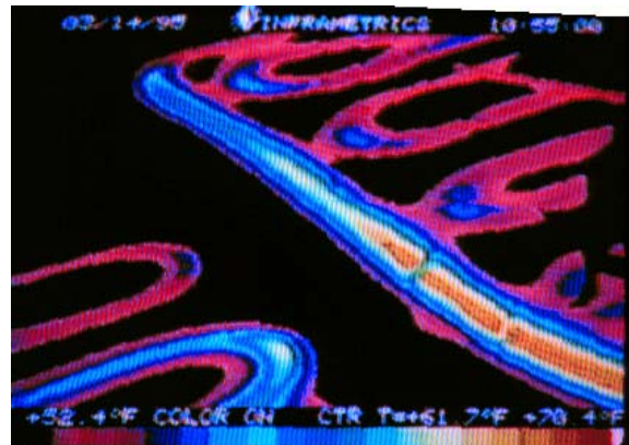
Image 8. Hydronic heating coils embedded in a concrete floor show up clearly in this thermal image.
