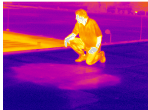
Image 10. The wet insulation in the roof system shows up clearly due to its greater thermal capacitance.
