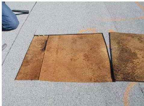
Figures 13, 14, and 15. Exploratory openings executed in roofing system to confirm roof composition, to validate results of infrared thermography study, and to determine actual location of moisture within the roof components.
